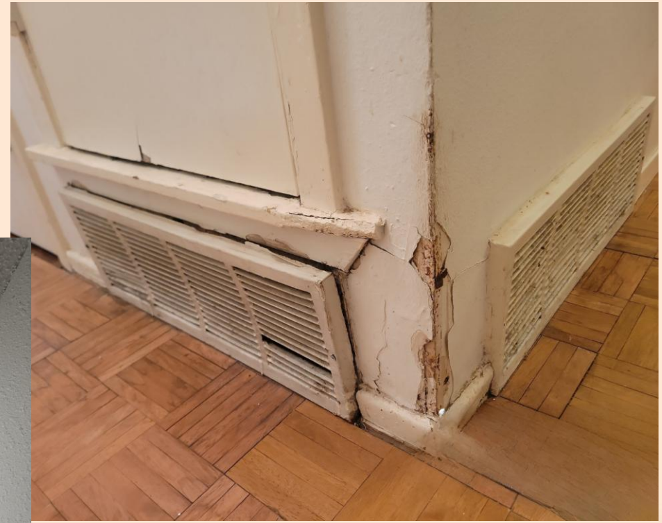
Interior wall damage
