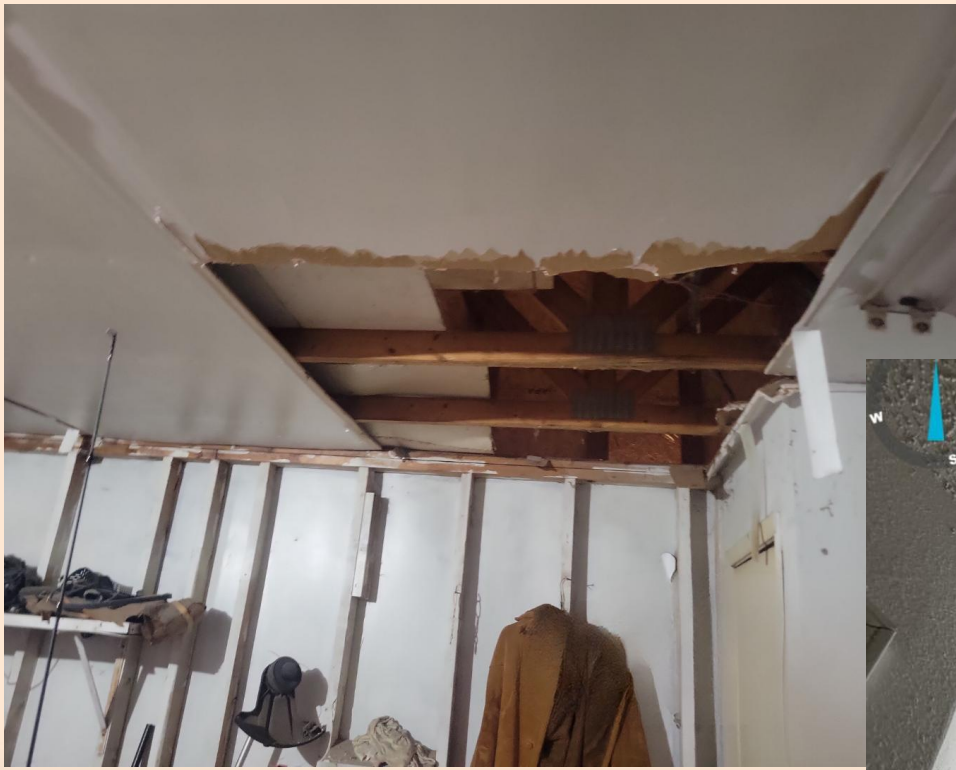
Missing garage ceiling - occupied
