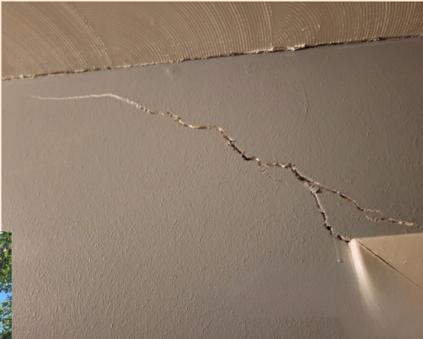
Wall cracking with separation
