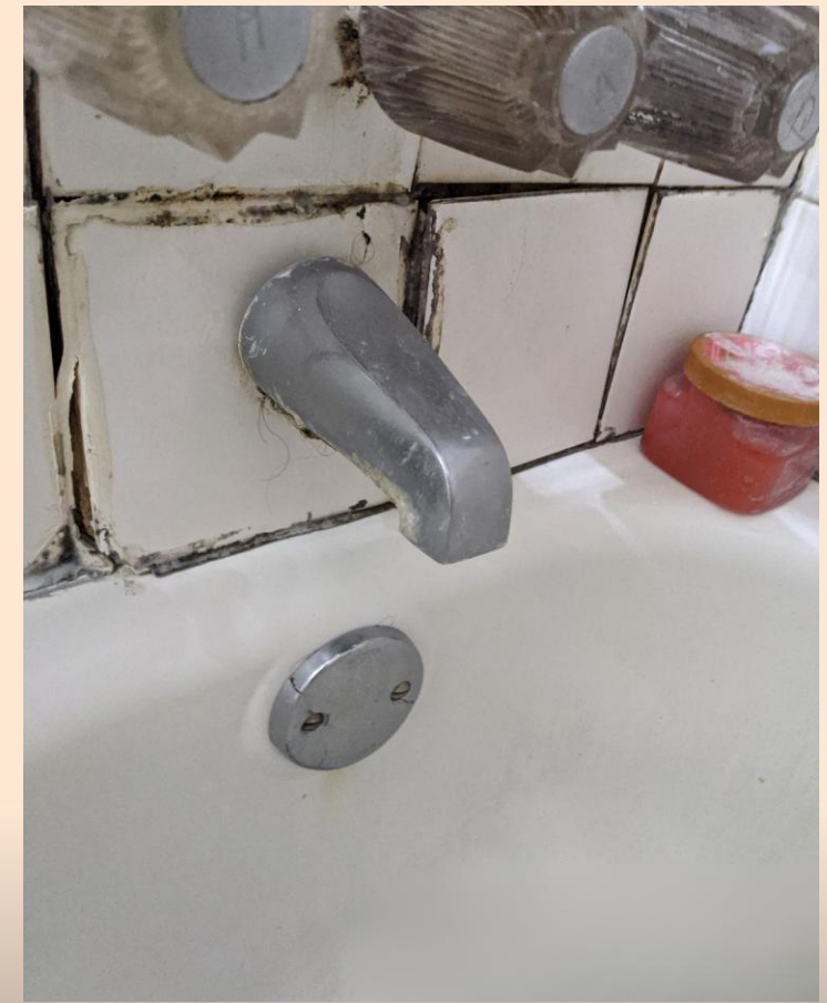
Damaged & Leaking tile - Occupied
