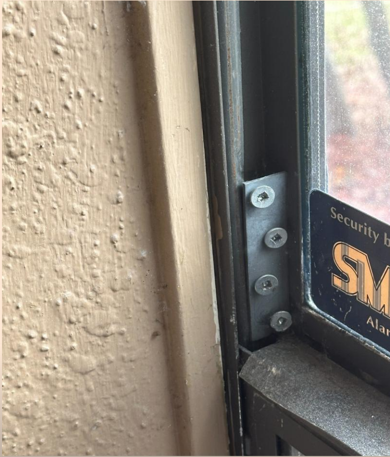
Window Sealed Shut
