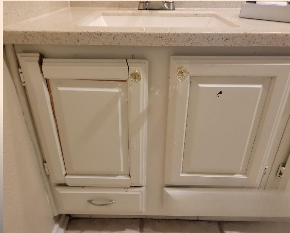
Damaged bathroom cabinet - "Move in Ready"
