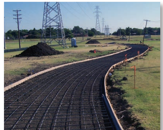
Progress continues on construction of Phase I of Heritage Trail, which consists of approximately 4.25 miles of concrete trails and sidewalks, three trailheads, major intersection enhancements, one exercise station, one pedestrian bridge and other improvements.
